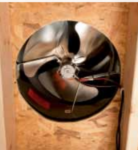
Roof Mount, Attic View
